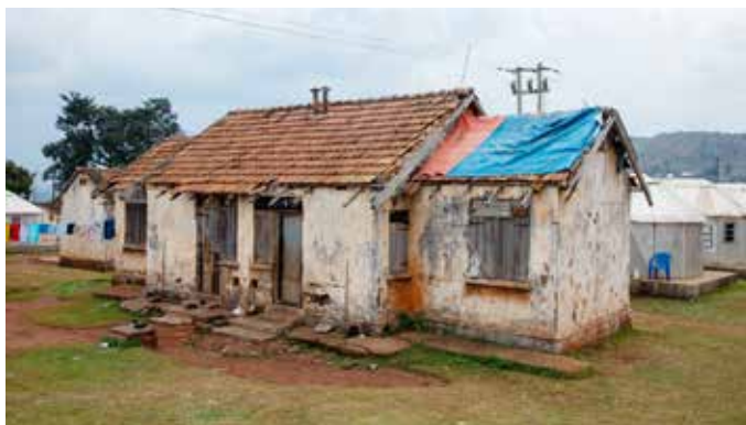
One of the outdated and poor state of housing units in some Police Barracks
